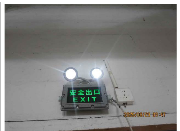
Test for emergency light
