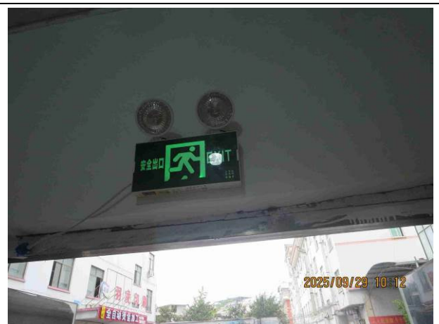
Safety exit sign and emergency light
