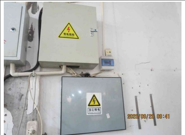
All the external covers of all electric boxes were locked
